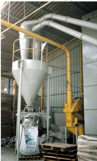
Pneumatic conveying to bagging equipment
